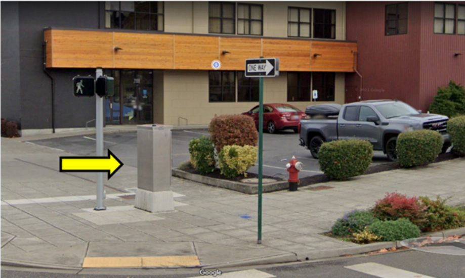
Figure 3-5. Signal Control Cabinet (State and Maple Sts, Bellingham, WA) 9
